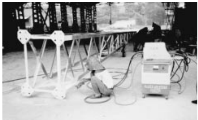
Fig. 2 Arc-sprayed Al coatings were applied to the steel tower for acid corrosion resistance
